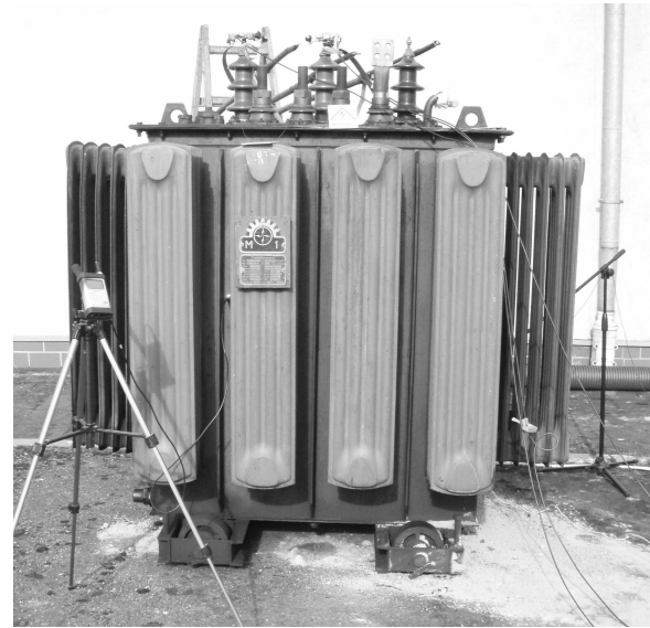
Fig. 12. Transformer TONa 800/15 0.8 MVA during recording of the tank vibration signal
